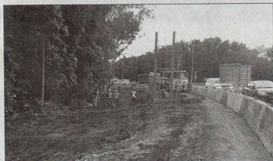
NLEX ADDS LANE AT SAN FERNANDO NORTHBOUND EXIT: NLEX Corp. is building a major lane at the San Fernando interchange northbound exit which is expected to be completed in March this year. It will address the heavy volume of vehicles in this area in Pampanga. The expansion project will widen the 336-meter northbound exit ramp heading towards Pampanga's capital city, increasing the number of lanes to two. A traffic management plan has been put in place around the work area to assure motorists and ensure convenient travel while construction is going on. NLEX is deploying traffic personnel to manage the traffic.
